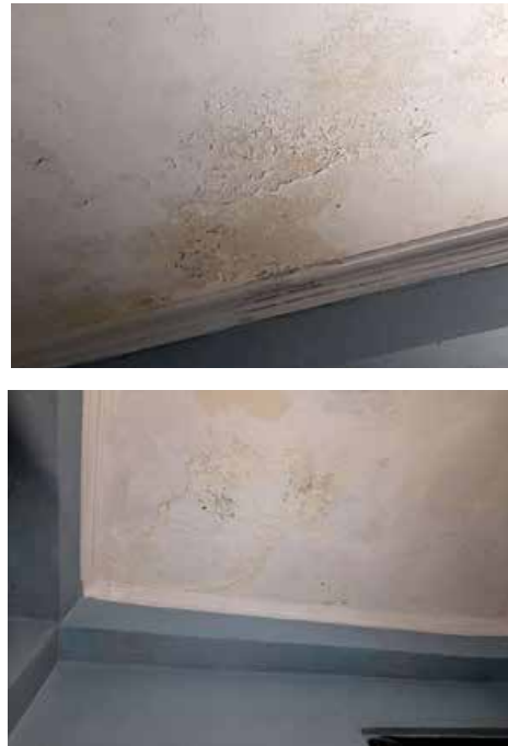
Fig 2 & 3 Show the penetration in roof
